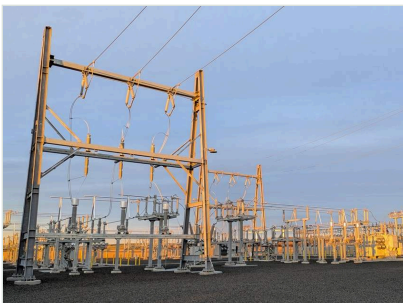
RAILROAD AVE 115 kV · COMMISSIONED 2025
