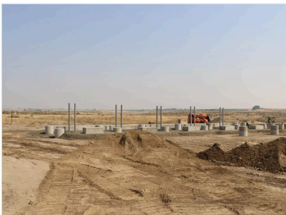
CAMP SUBSTATION · OWNER'S ENGINEER, 2024-26
